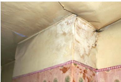
▲ Internal penetrating damp
