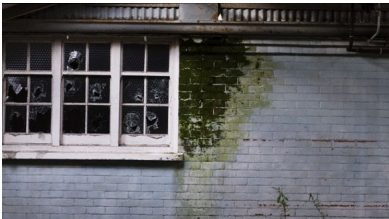
▲ Penetrating damp becomes more noticeable when it rains
