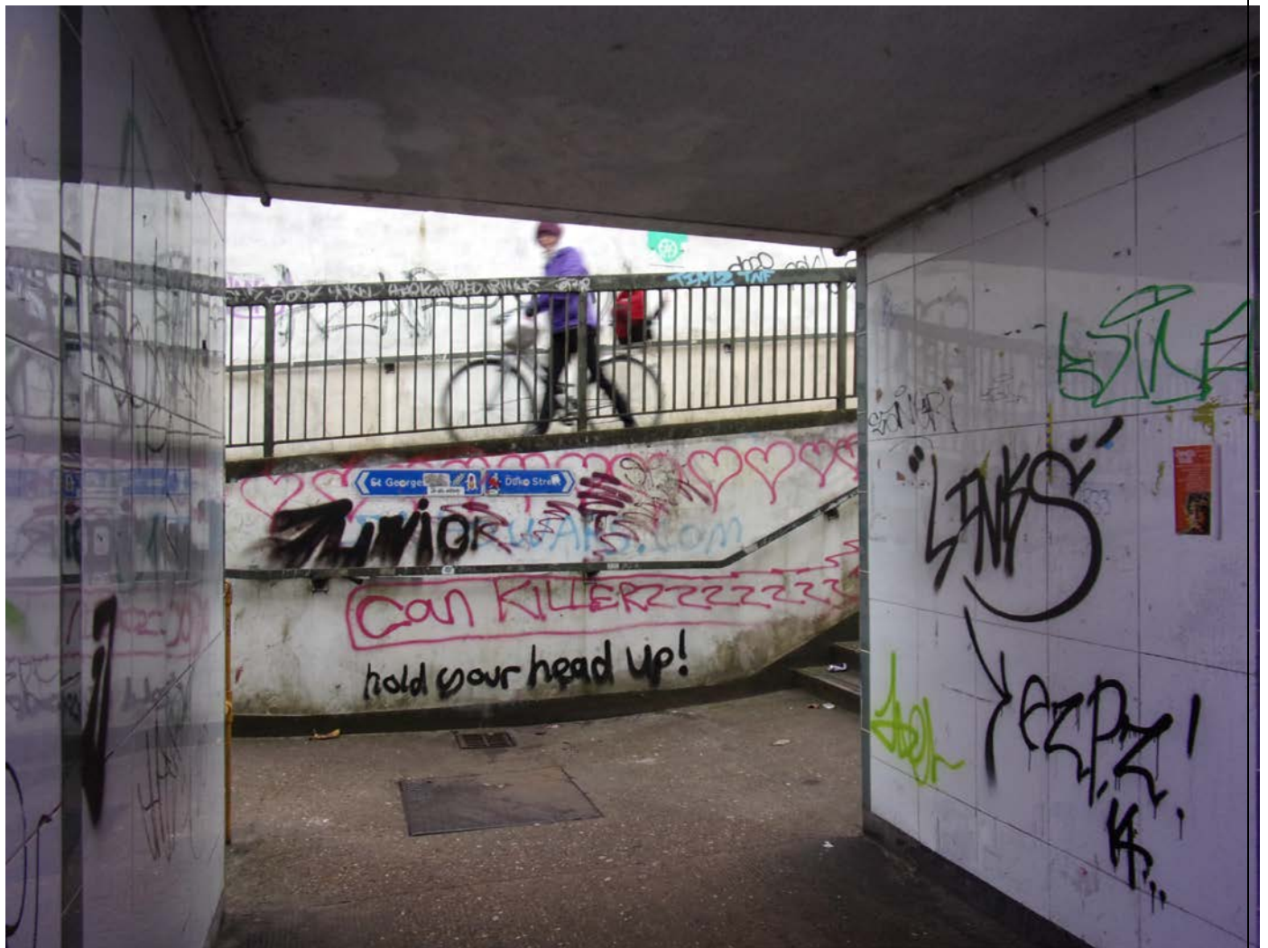
St Crispins subway – proposed for replacement as part of the new programme
