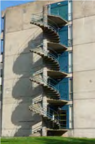
Above: 'Temporary' spiral staircases show where the Teaching Wall was intended to be extended.
