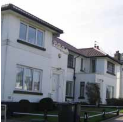
Fig 39: Bracondale Court (1937) with inappropriately replaced windows and door on the left and original windows on the right.
