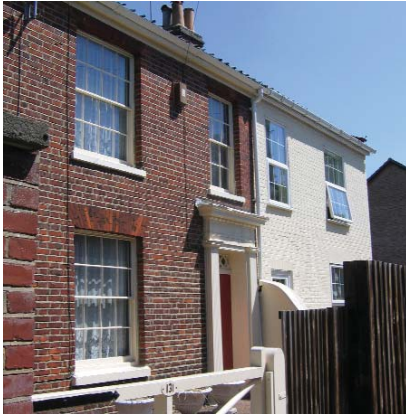
Loss of architectural details can significantly change the appearance of a building.
