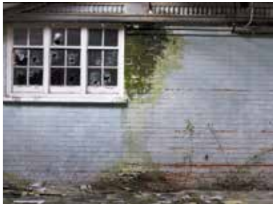
▲ Penetrating damp becomes more noticeable when it rains
