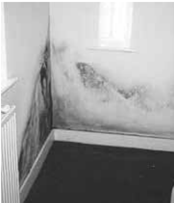
▲ Walls with black mould growth
