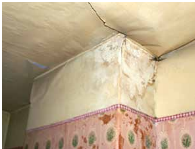
▲ Internal penetrating damp
